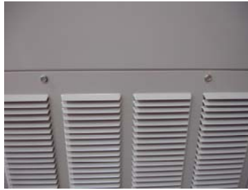
Figure 13 – Inlet grill of Air Conditioner
